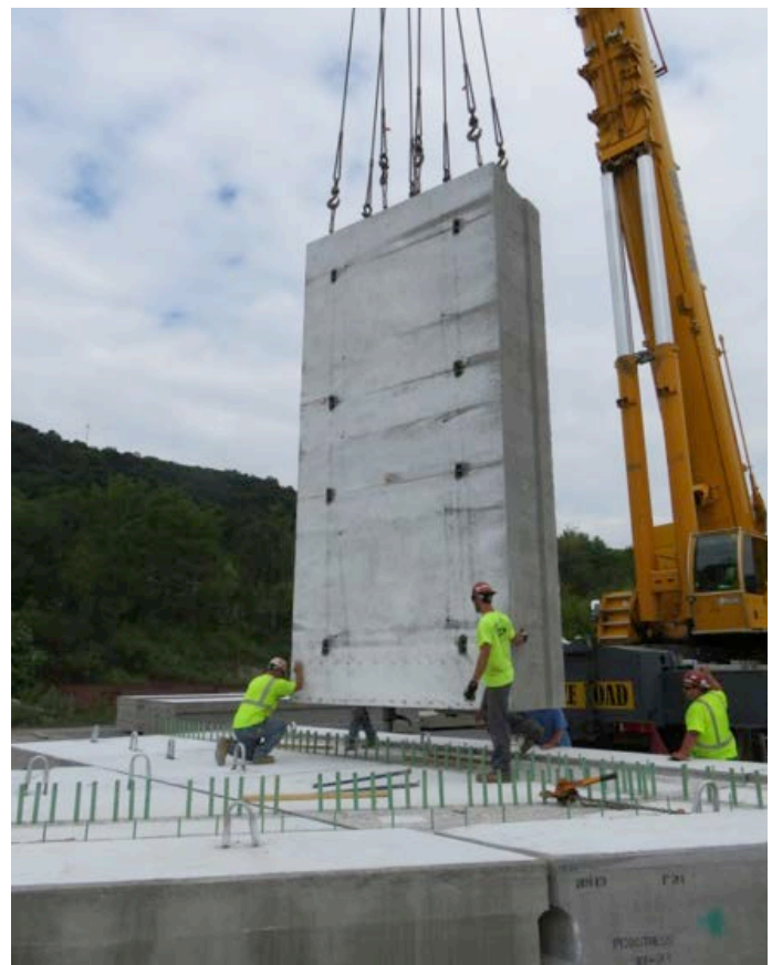
Dry fitting bridge components at PENNSTRESS' plant ensured a smooth operation on site.
